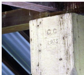
Condition of a post dated 1933. The painted rendered masonry posts replaced the original timber posts.
