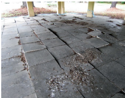
The existing condition of the concrete pavement. The paving is not original, is uneven, with evident displacement of some of the concrete pavers. Damage is likely the result of the overgrowth of adjacent mature tree's roots.
