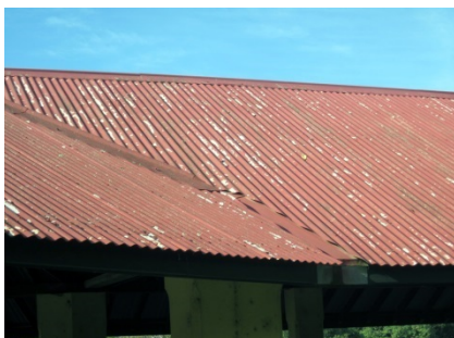
The existing condition of the corrugated iron roof sheeting. There is some damage to the paint finish and roof sheets.
