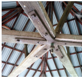
The existing condition of the roof structure. There are some missing elements and damage to the vertical steel tie rod and connection plate.
