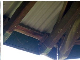
Damage to a timber fascia board.
