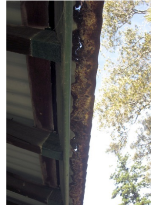
An example of corroded sections of roof sheeting.
