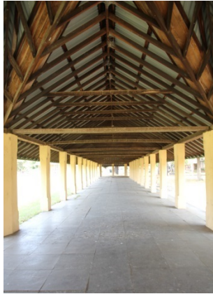
The interior of the former Shelter Shed showing the timber roof and support post structure. Two of the masonry posts have excessive leans and will likely need to be replaced. Much of the timber is not original.
