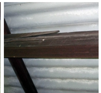
Splits and damage to original and non-original timber.
