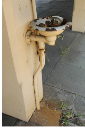
The existing condition of the water bubbler. The bubbler is corroded and there is damage to the paint finish.
