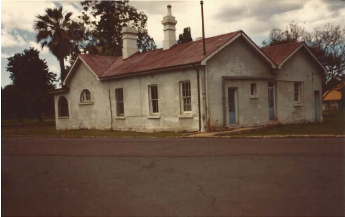
C-12 A 1975 photograph of the north and west elevations of Pine Cottage. Source: Terry Smith
